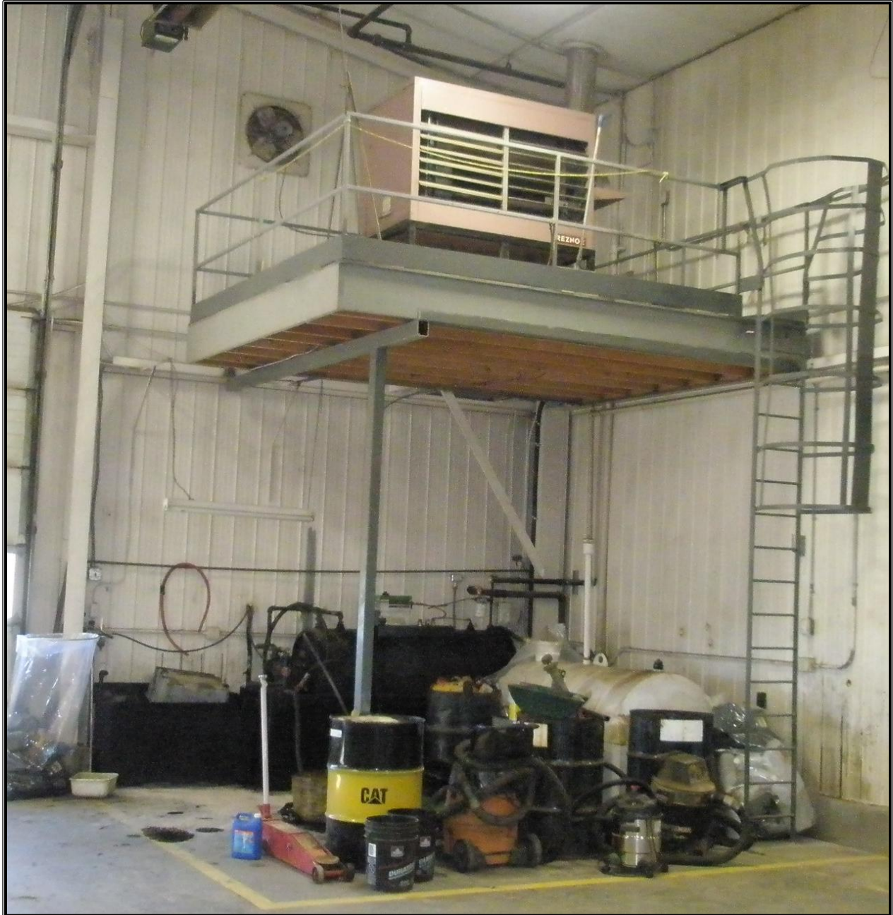
Figure 3-6 Reznor Waste Oil Heater at the County Shop
